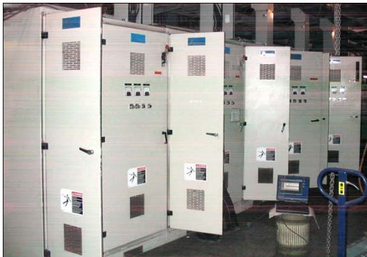
Figure 2 – New Drives in Attic Line-Up
